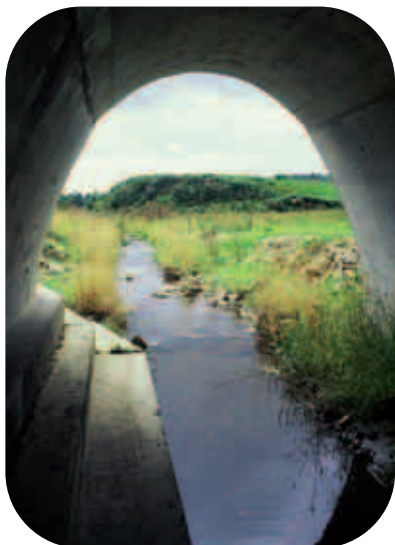
Artificial waterway for otters on motorway A89
