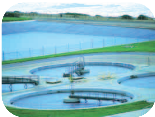
Wastewater treatment plant in Bolivar, benefiting from a replanting programme in the surrounding forest area, Adelaide, Australia
